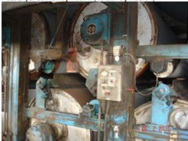
Post Dryer section by Toschi (10 Bar Cylinders!!)
