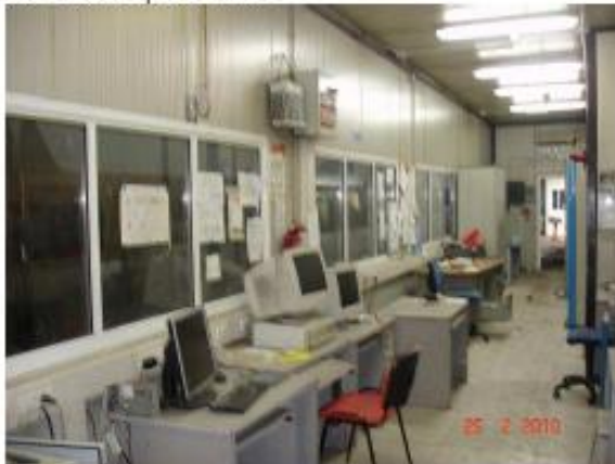
Main control panel room
