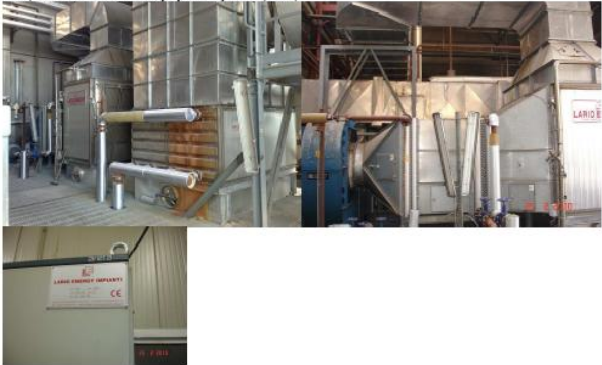
Complete New Heat recovery system by Lario (2005)
