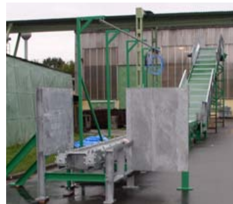
Illustrative photo: outgoing chain-belt conveyor
